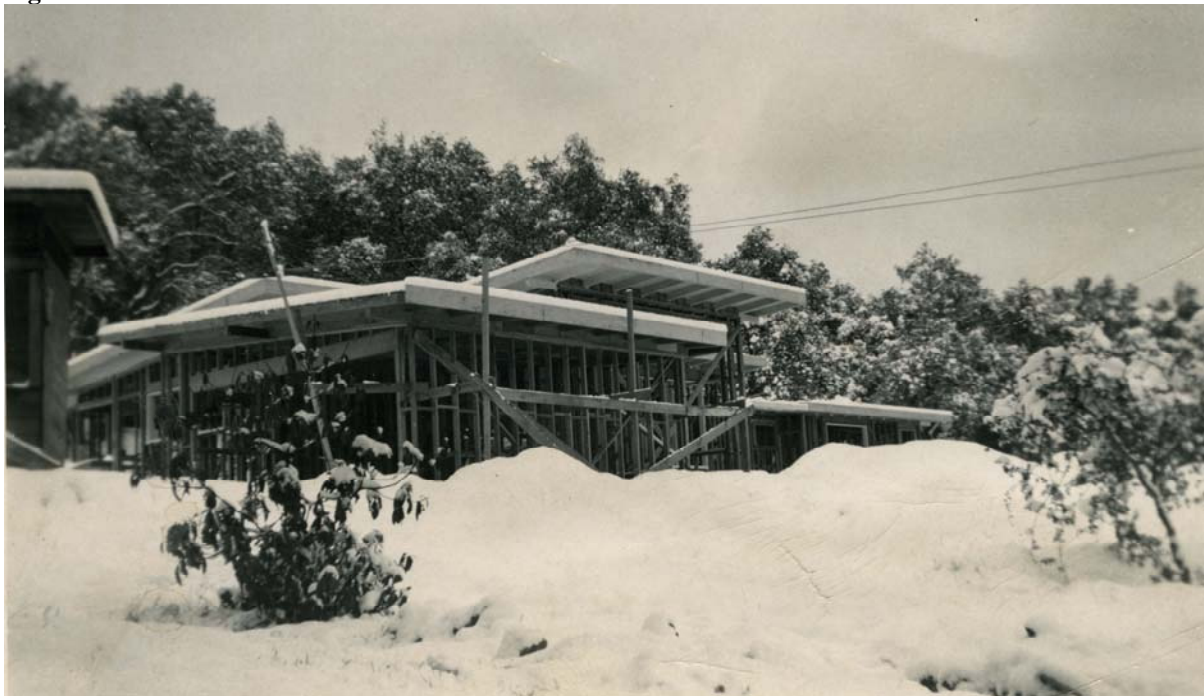
Photograph of house under construction, view facing southwest, 1949, courtesy of Theodore Thomas, Jr.
